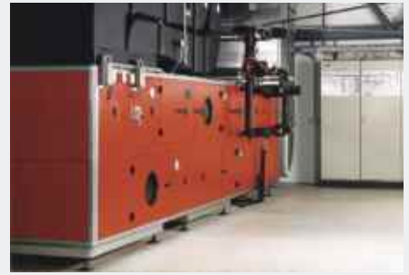
HVAC system installed in cellar
