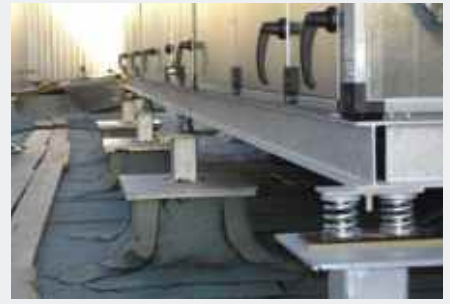
Roof-mounted HVAC system
