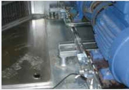
Bearing of belt-driven fans
