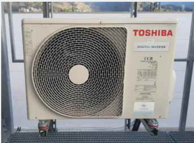
External air conditioning unit on wall bracket
