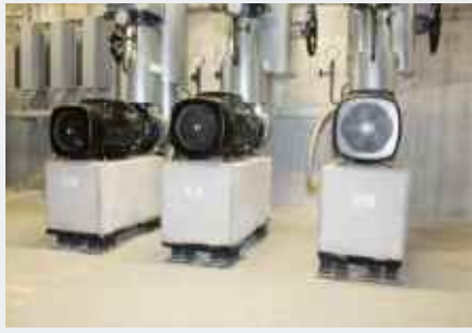
Bearing of pumps with additional mass
