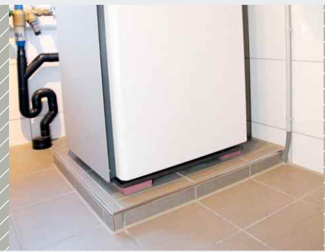
Sylomer® discrete bearings for a heat pump
